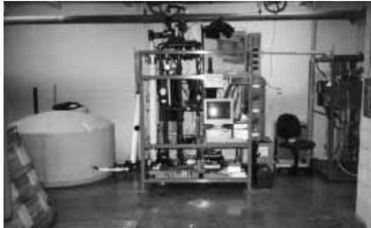
Figure 4-11 COMFOWARD System in Decatur, Illinois
