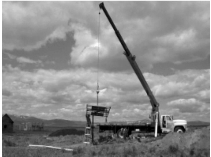
This PV array was assembled and wired on the ground, then lifted with a crane.
