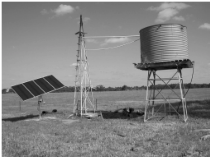
Windmill replacement in the Australian Outback Installation by BW Solar (Perth, Australia)
